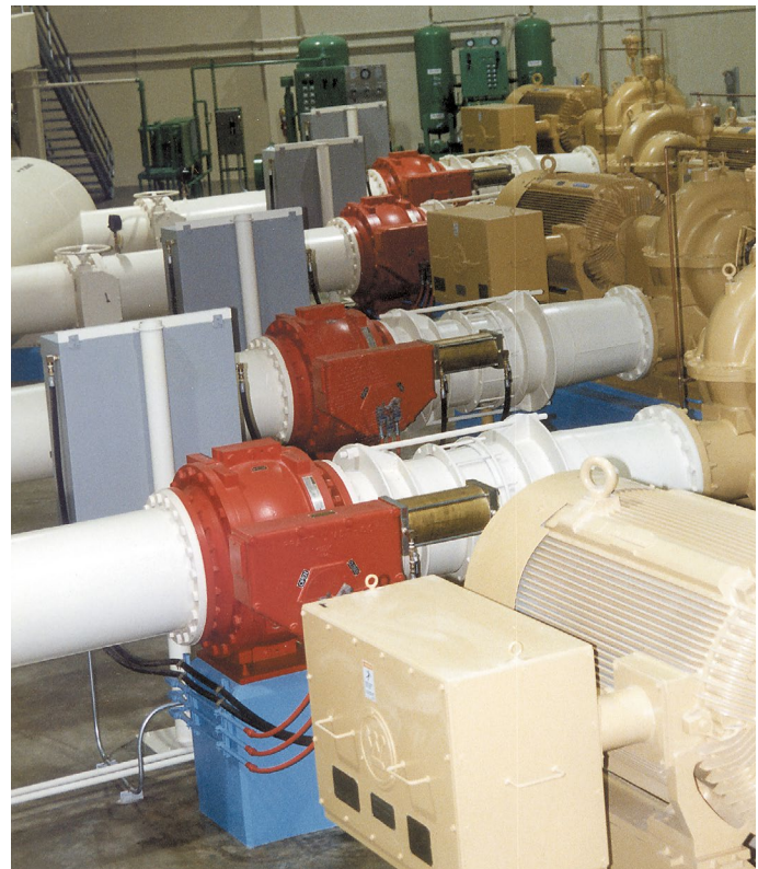
20" METAL SEATED BALL VALVES IN PUMP CONTROL SERVICE
